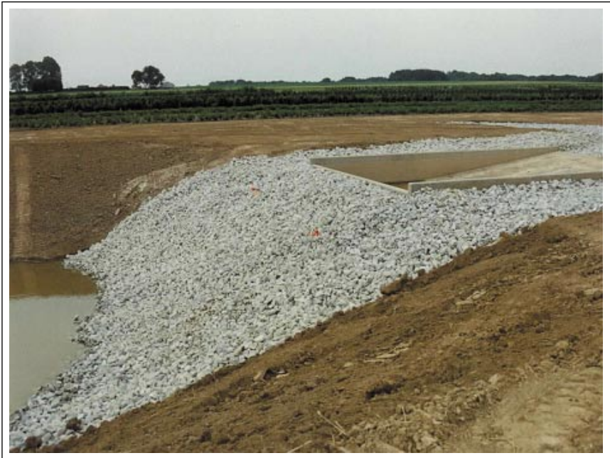
Figure 2. Rock layer on the surface of the pond wall below the weir.
